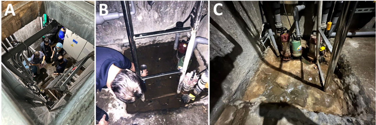
Figure 2. Basement mechanical area in an investigation of a fatal case of Naegleria fowleri primary amebic meningoencephalitis from indoor surfing center, Taiwan, 2023. A) The opening to the basement with ladder visible to right of opening; B) stagnant water beneath the basement ladder; C) depression under basement ladder after water was drained.
